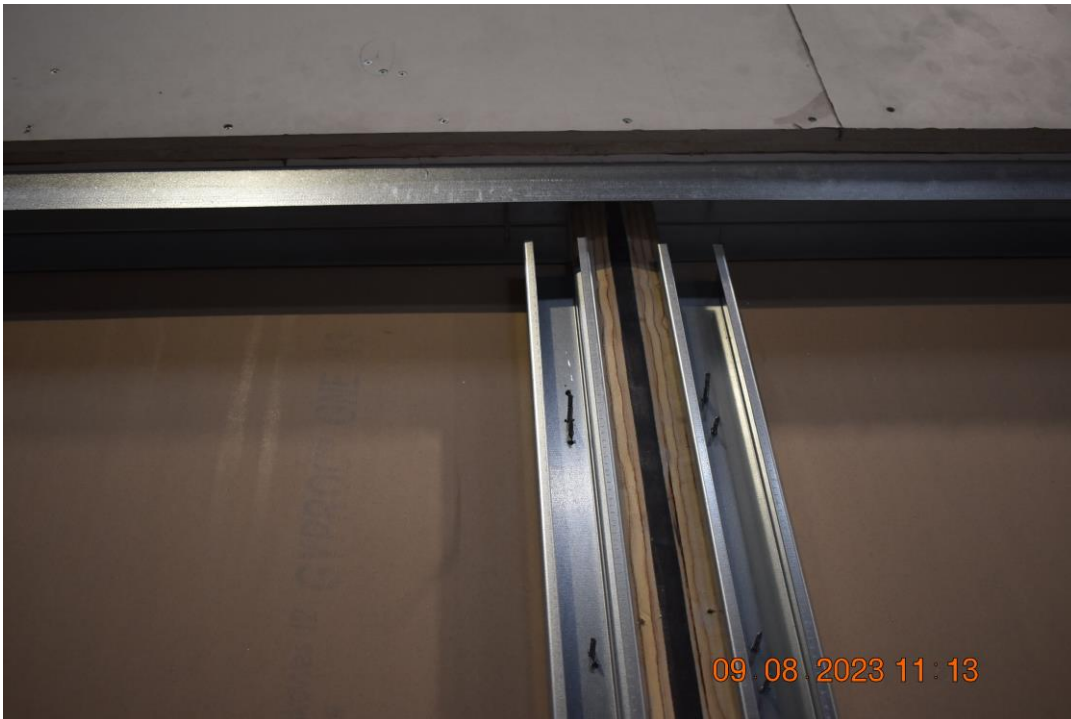
Photo No. 8 Prefabricated tongue and groove system, seen from inside the wall, connected to the fixed wall system.
