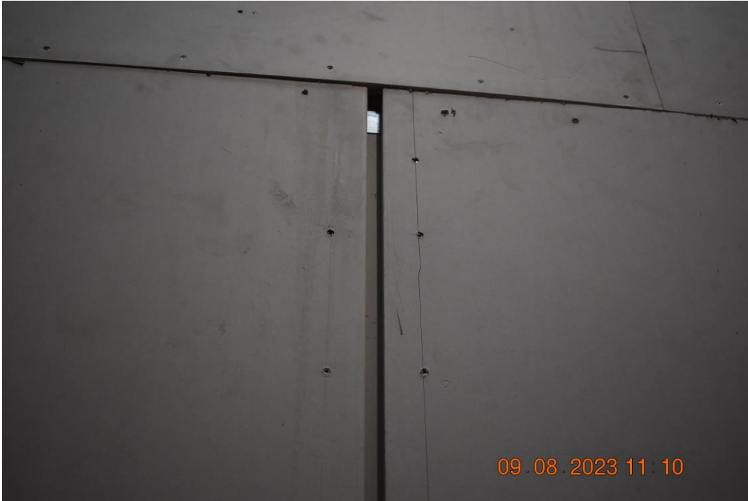
Photo No. 7 Prefabricated tongue and groove system, seen from outside the wall, connected to the fixed wall system.
