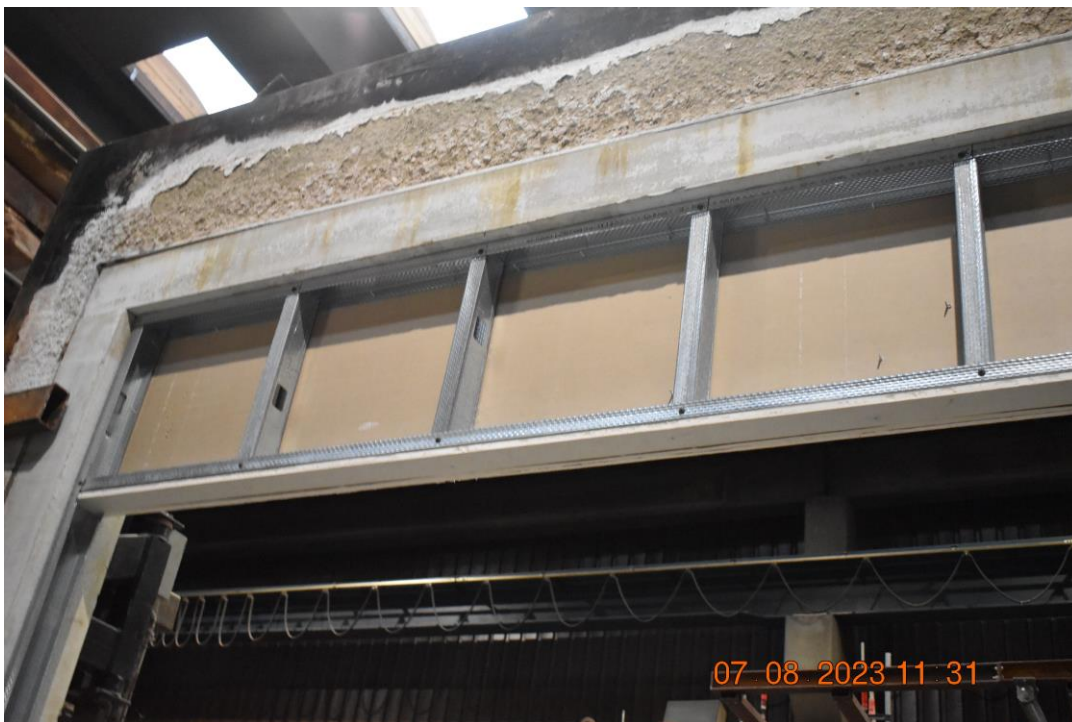
Photo No. 2 Fixed steel framework panel frame mounted with gypsum on one side and bottom.
