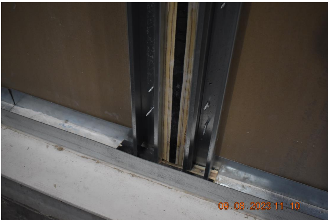
Photo No. 6 Prefabricated tongue and groove system, seen from inside the wall.
